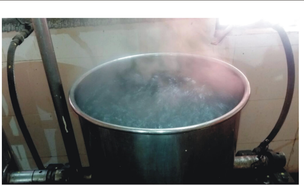
Hot Water for Girls using Solar Thermal
